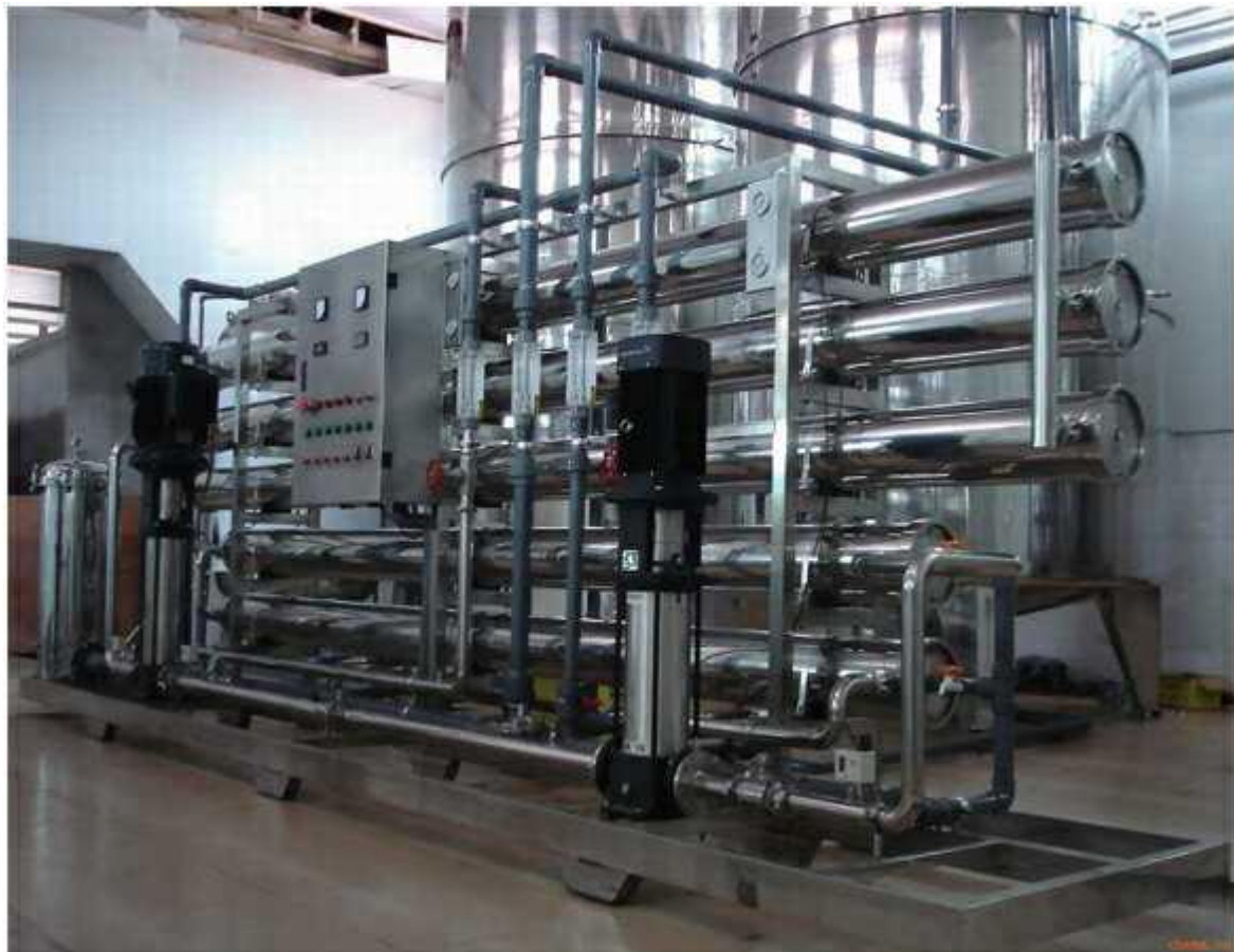
某食品厂 40 吨纯水装置 40 ton pure water plant of a food factory
